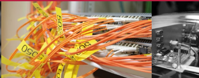
Network cables (fiber optic)
