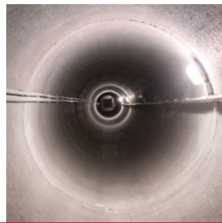
View from the inside of the underground heat collector for the external air supply at the Environmental Campus Birkenfeld
