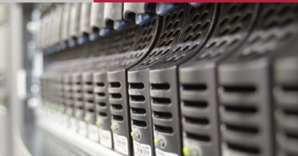
Detail view of server
