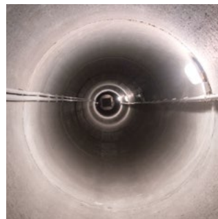
View from the inside of the underground heat collector for the external air supply at the Environmental Campus Birkenfeld
