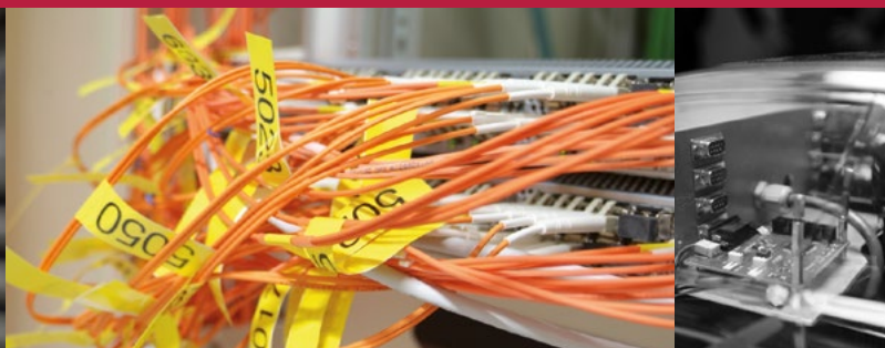
Network cables (fiber optic)
