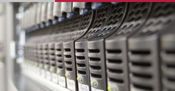
Detail view of server
